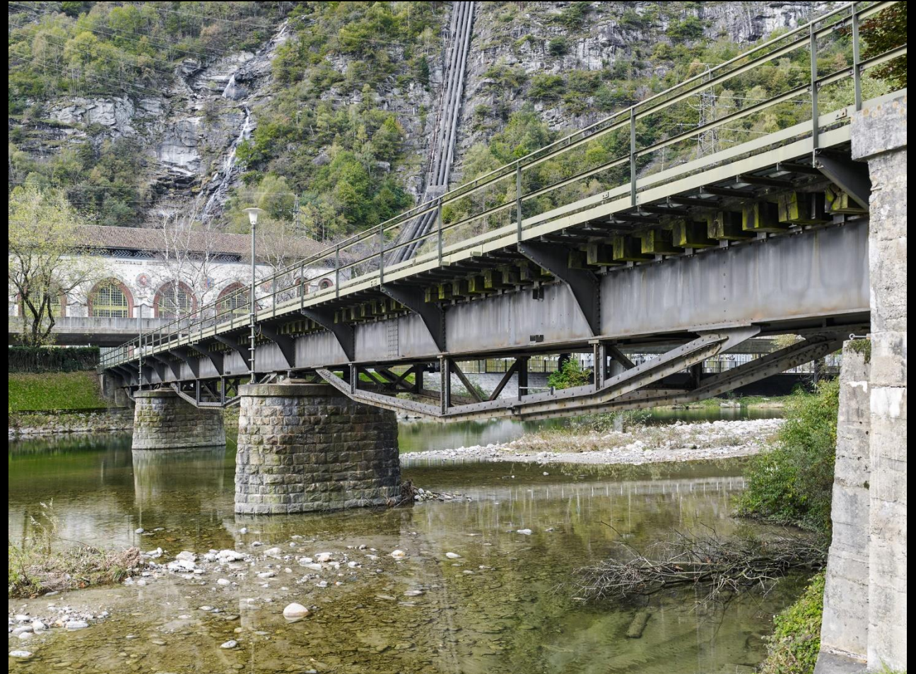
Example: Steel superstructure on stone masonry piers, concrete abutments (Ticino Bridge Atel, photo © Georg Aerni)
