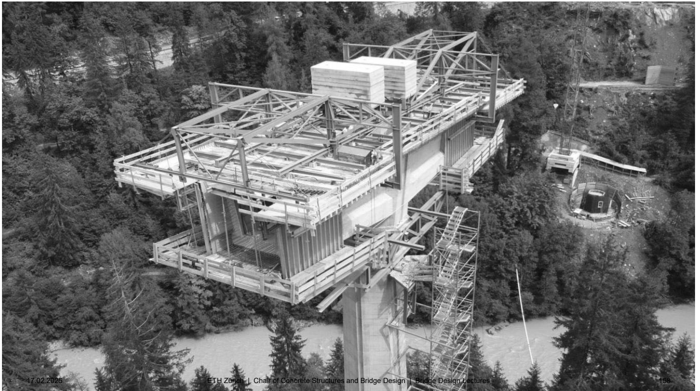
Balanced cantilevering, basic section (length given by dimensions of the two free cantilevering carriages).
