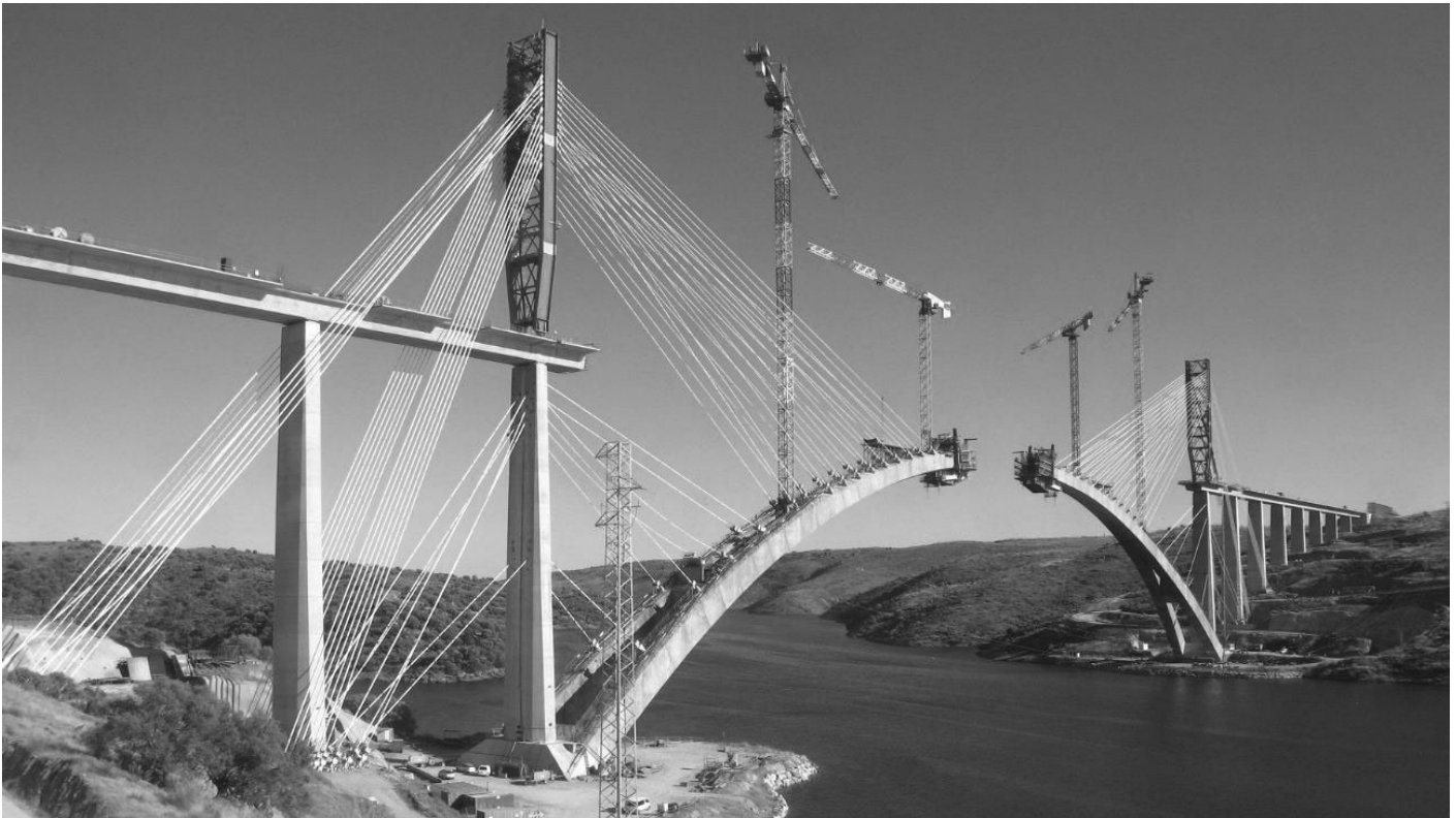
Photos: Viaducto de Almonte, Arenas & Asociados (J.J. Arenas, G. Capellán, M. Sacristán), High Speed Line Madrid-Extremadura-portugal, Cáceres, Spain (2016). High speed train concrete deck arch bridge, main span 384 m, total length 996 m, f/L = 1/5.7 . Hollow box high strength concrete arch, prestressed concrete box girder.
