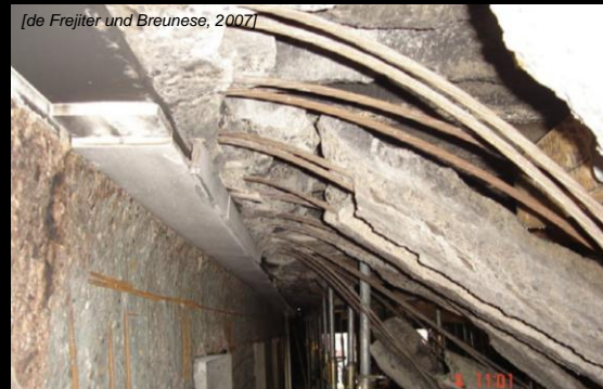
Fire in underground parking, Rotterdam (2007)
