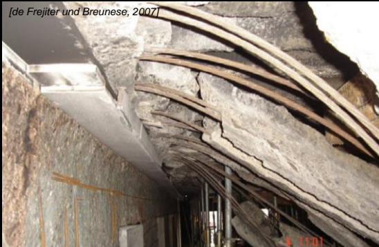
Fire in underground car parking, Rotterdam (2007)
