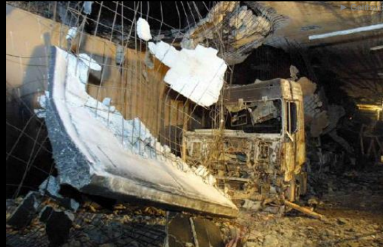
Suspended ceiling with severe damages over a length of around 230 m
