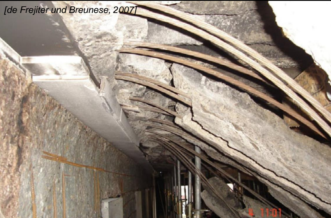
Fire in underground car parking, Rotterdam (2007)
