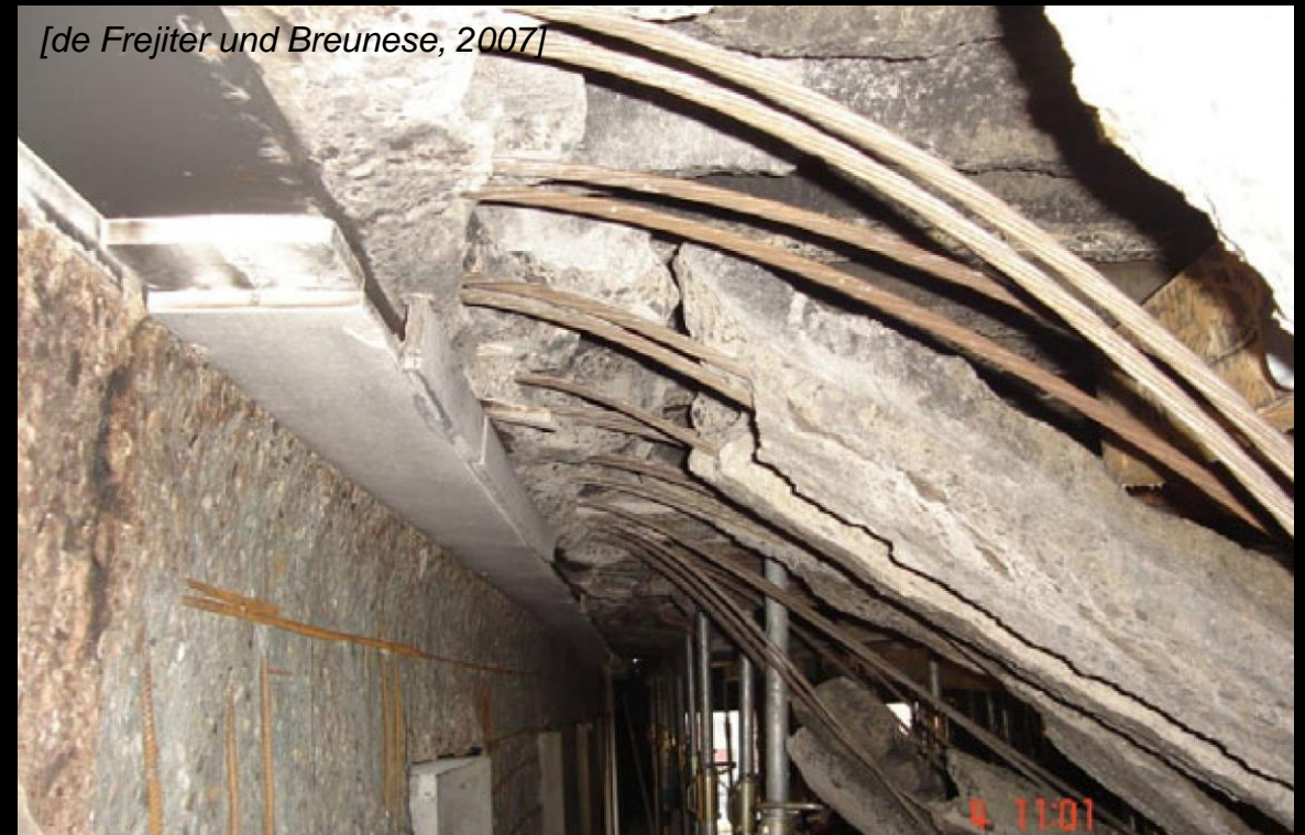
Fire in underground parking, Rotterdam (2007)
