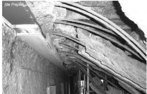
Fire in underground parking, Rotterdam (2007)
