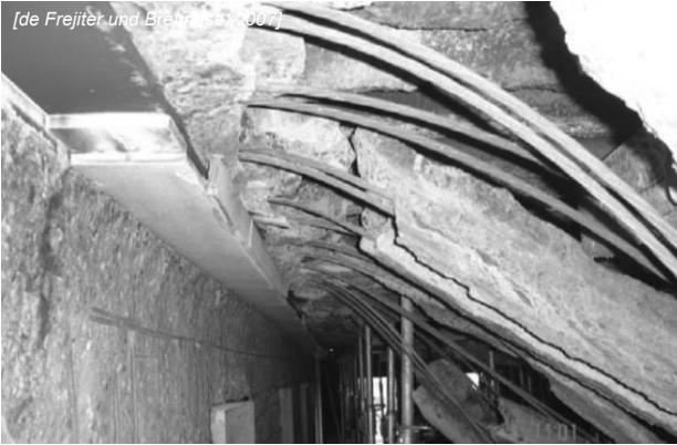
Fire in underground car parking, Rotterdam (2007)
