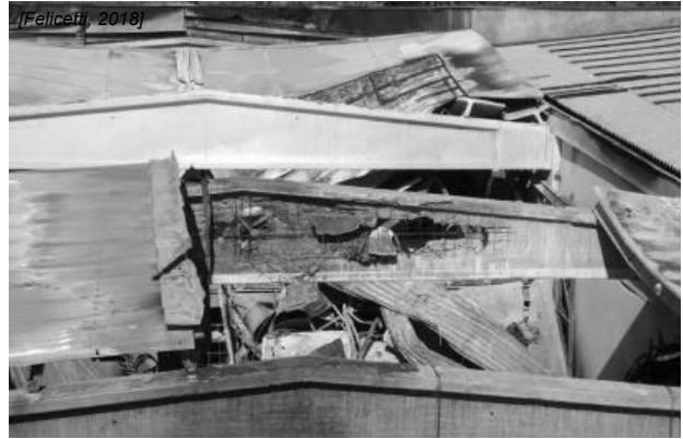
Fire in warehouse, near Milano (2018)
