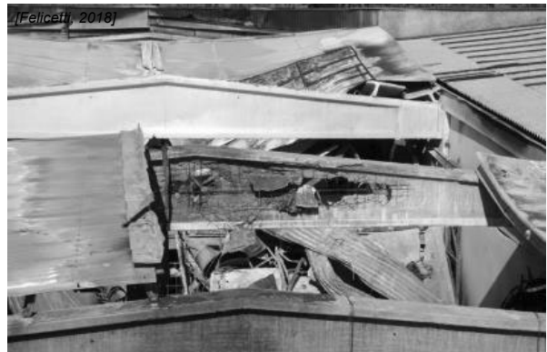
Fire in warehouse, near Milano (2018)
