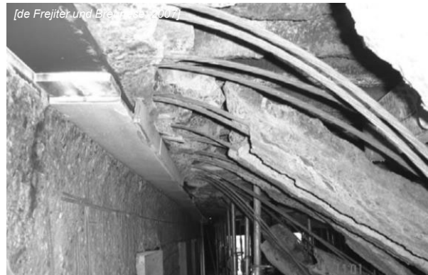
Fire in underground parking, Rotterdam (2007)
