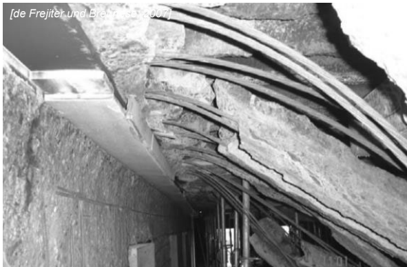
Fire in underground car parking, Rotterdam (2007)
